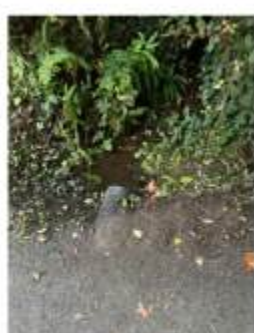
B5. Direct Discharge Point from Lacamas Shores (1 of 35): constant water flow
